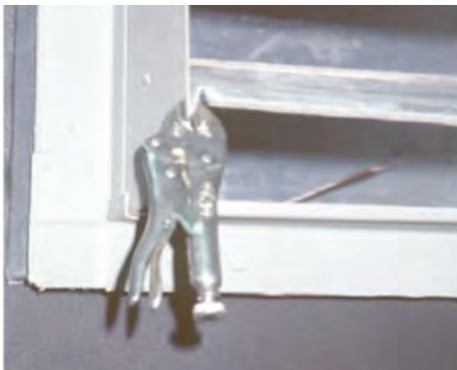
Figure 9.7.2. Damper quick fix – not recommended
