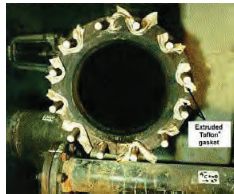
Figure 9.3.8. Failed gasket on blind flange
