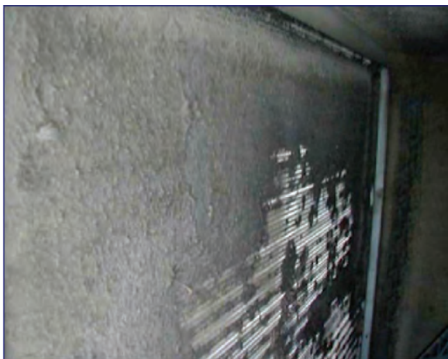
Figure 9.7.1. Cooling coil requiring cleaning
